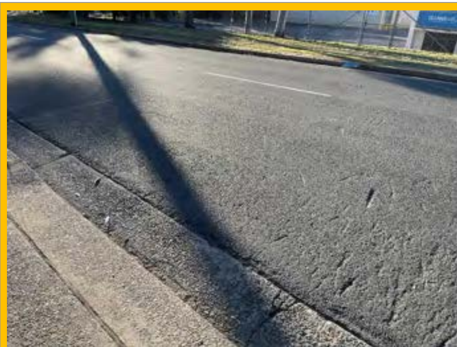
No. 033: gouge marks at 8 Harris St
