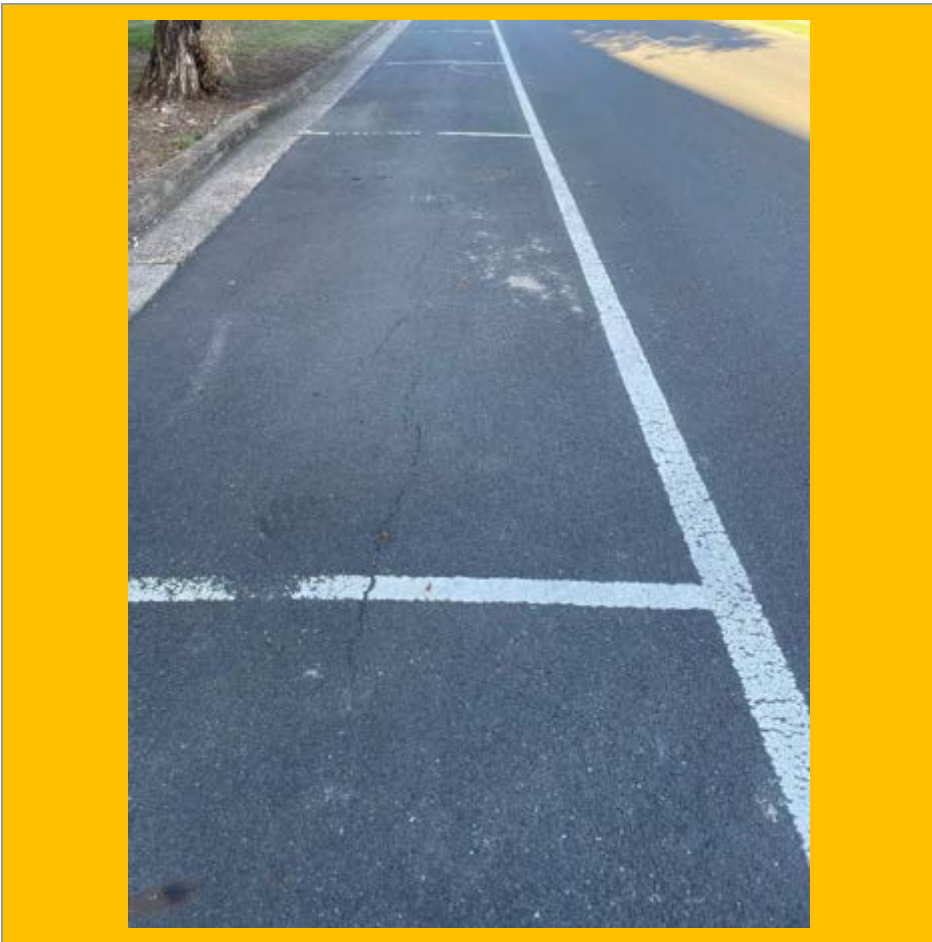
No. 025: Longitudinal cracking in road surface from approx. 135m to 140m
