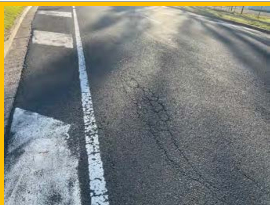
No. 046: cracking and deterioration of road surface from 210m to approx. 217m
