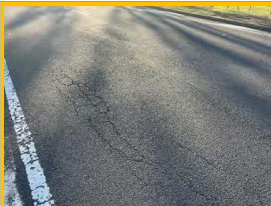
No. 045: cracking and deterioration of road surface from 210m to approx. 217m
