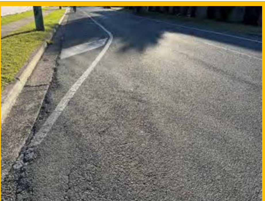
No. 096: 370m. deterioration to road surface radiating west from car park entrance
