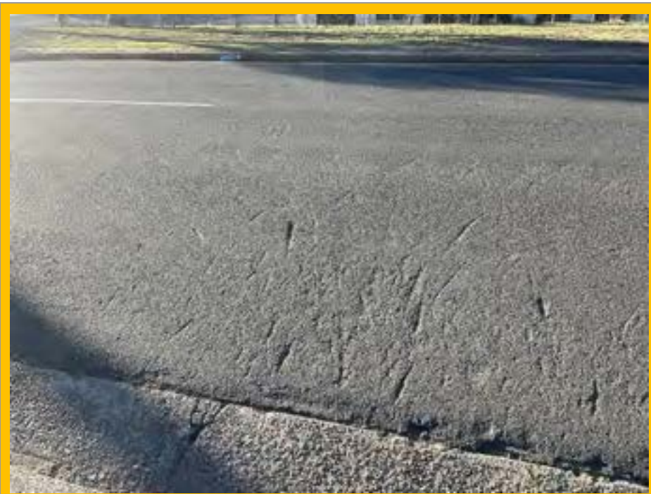
No. 032: gouge marks at 8 Harris St
