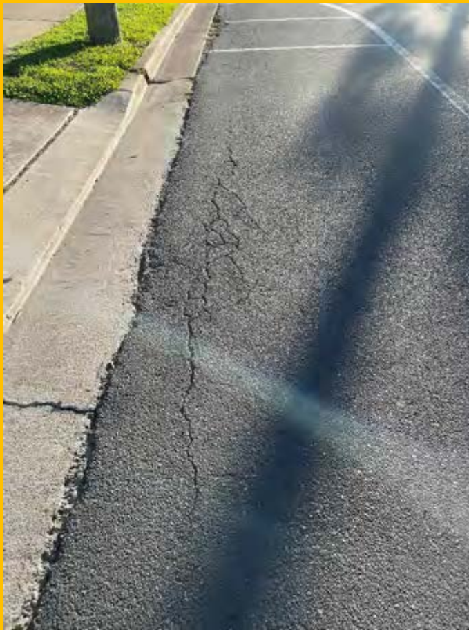
No. 057: cracking and deterioration of road surface at western layback to 14-16 Harris St
