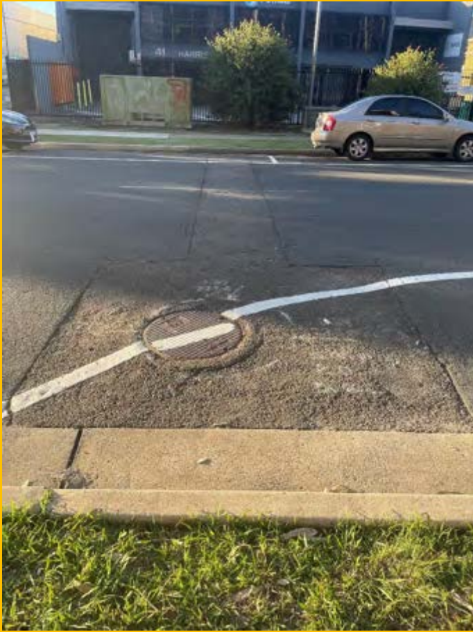
No. 115: depressions and cracking in road surface repairs extending across full width of road at 472m
