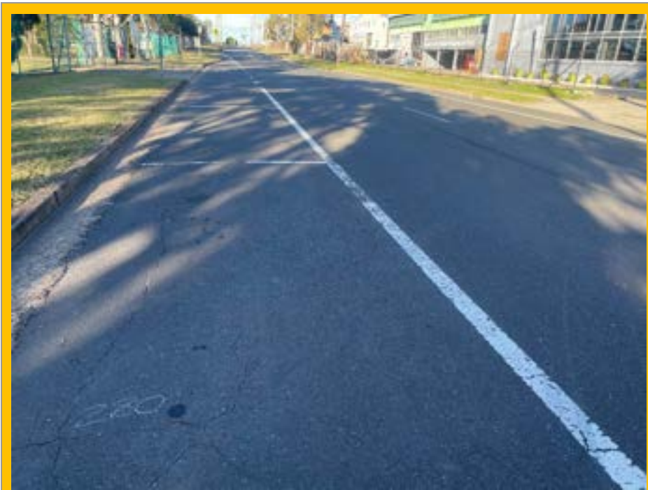
No. 051: 280m. Cracking in surface from approx. 279m to 283m
