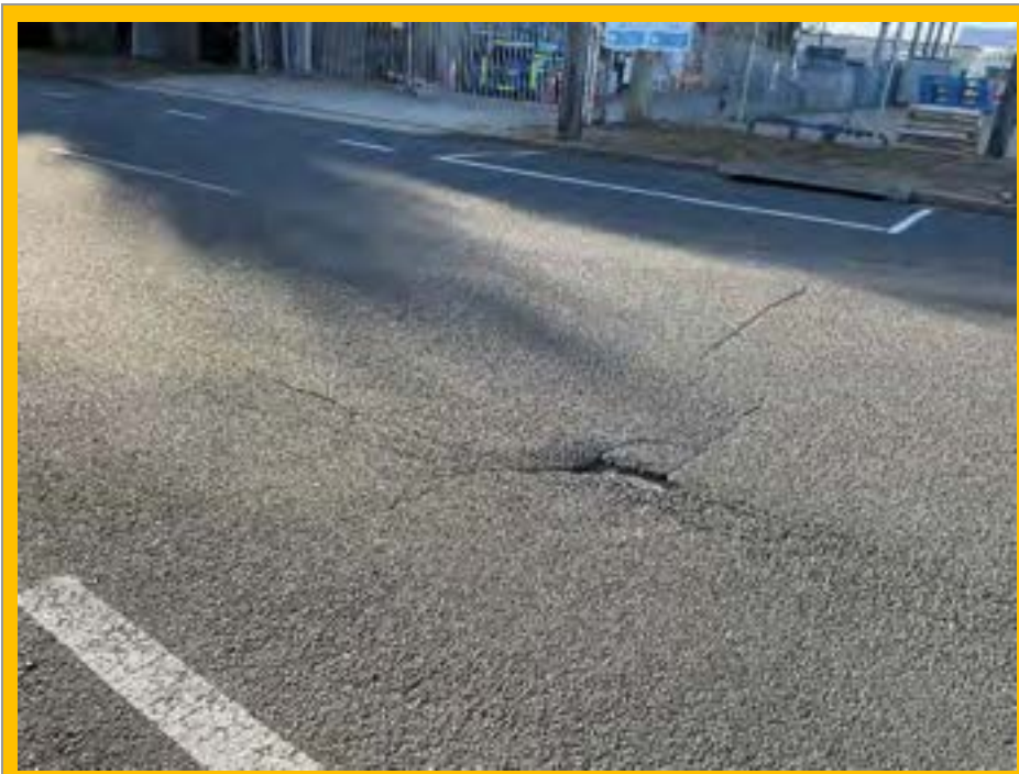
No. 091: damage and surface cracks at 355m
