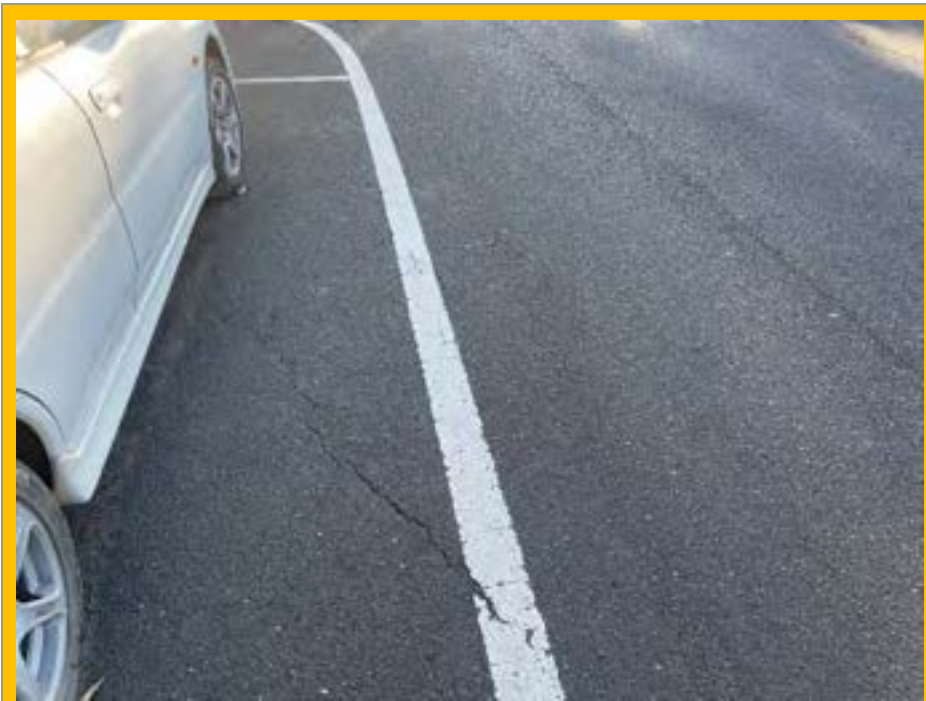
No. 113: continuation of crack in parking bay road surface at approx. 465m
