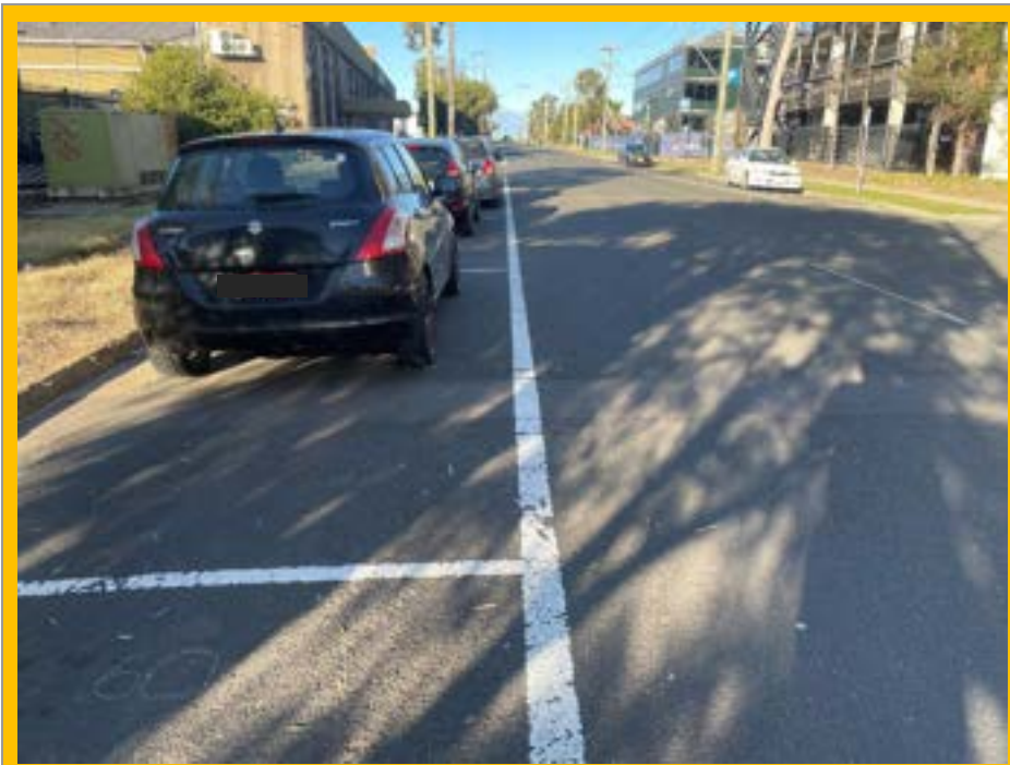
No. 013: 60m. Repairs to road surface across width of street at approx. 62m
