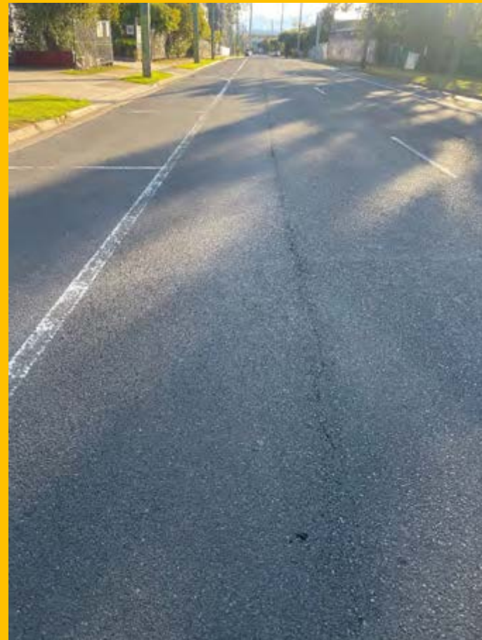
No. 052: longitudinal crack in road centre at join in materials commences from approx. 240m and continues through to approx. 290m
