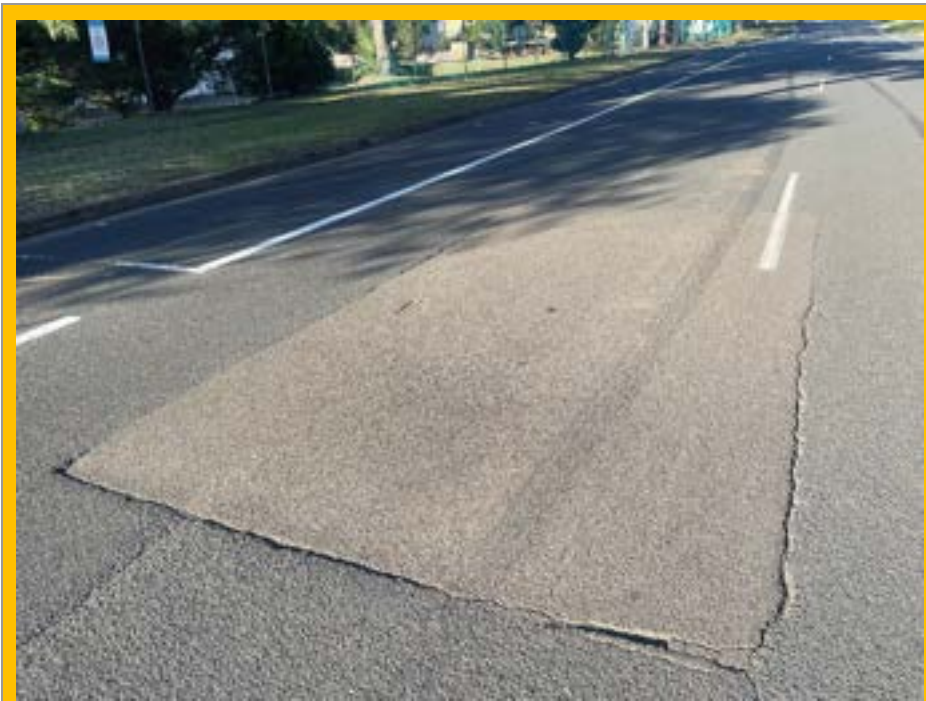
No. 047: cracking at repair to road surface from 261m to 265m
