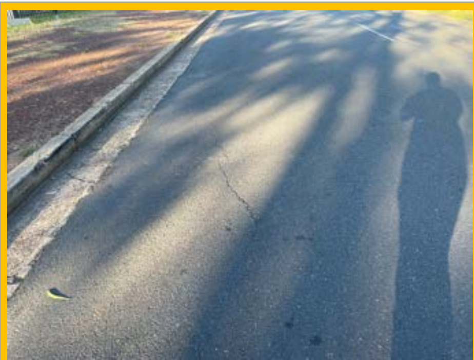
No. 079: cracking in road surface at approx. 456m
