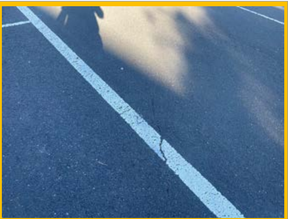
No. 030: Cracking in road surface at approx. 163m
