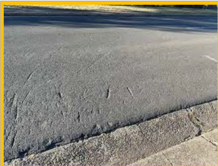
No. 031: gouge marks at 8 Harris St
