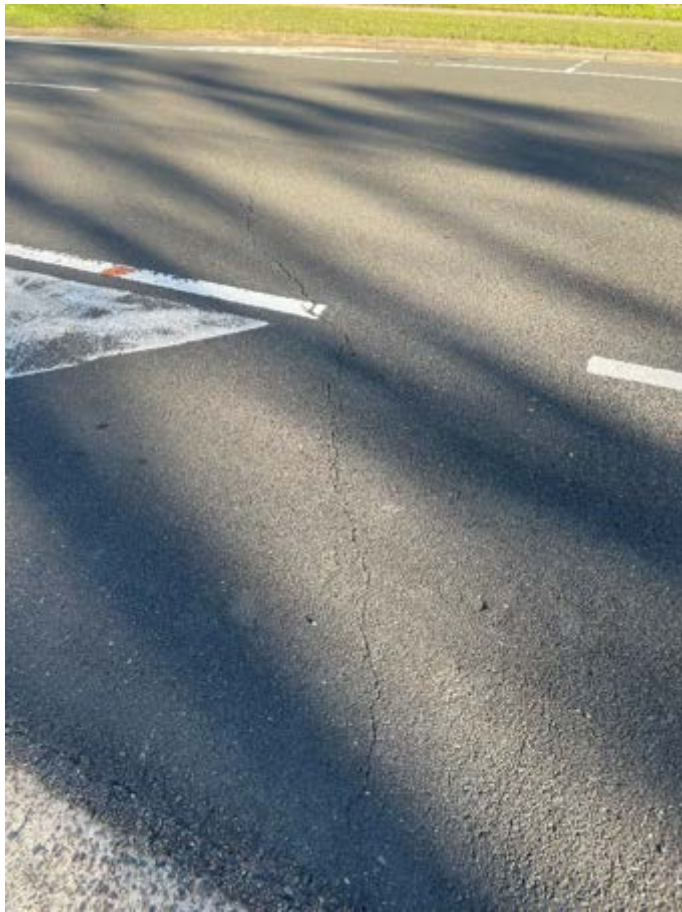
No. 061: lateral cracking from kerbline to centre of road at approx. 323m
