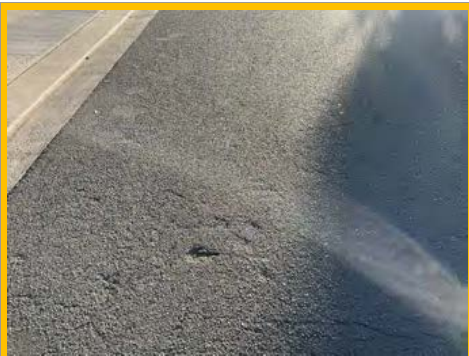
No. 117: gouging to road surface at 476m
