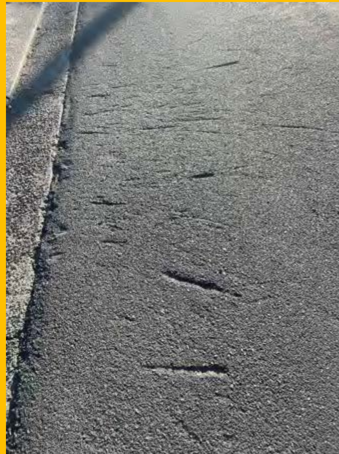
No. 030: gouge marks at 8 Harris St
