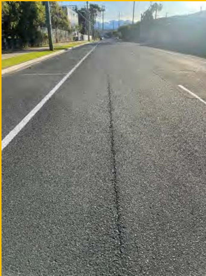
No. 069: continuation of crack in road centre
