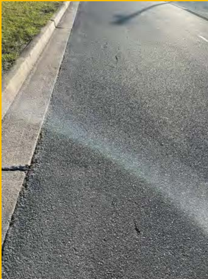
No. 009: gouge marks at 45-50m
