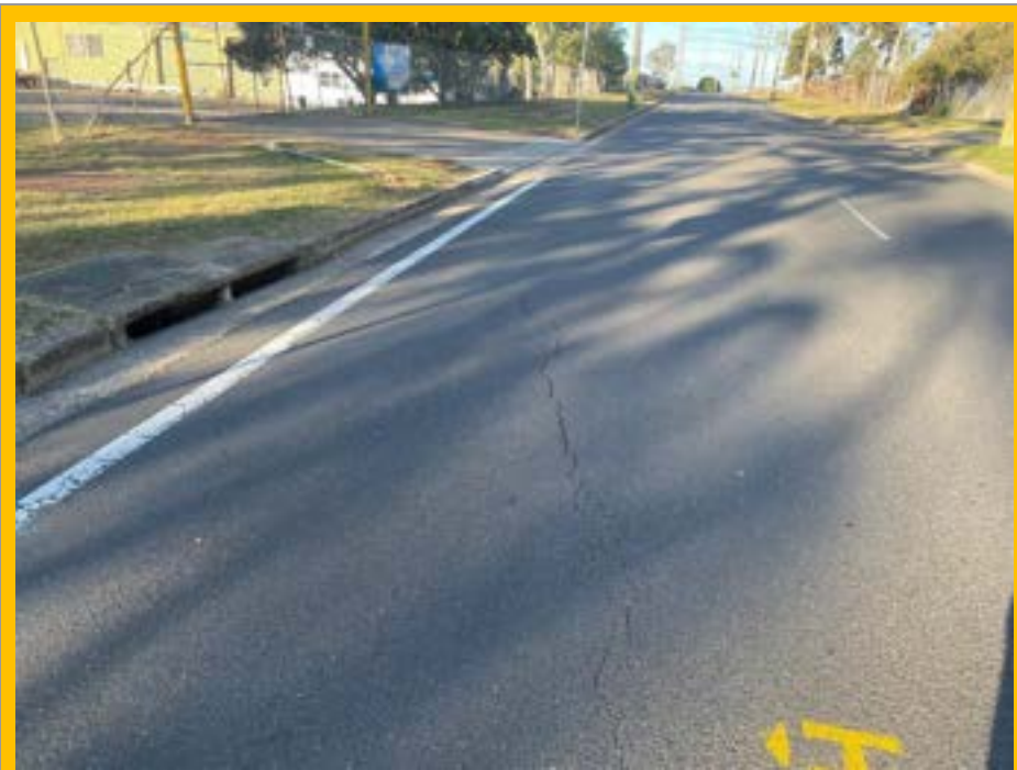
No. 064: cracking from centre of road leading toward kerblines at approx. 344m to 352m
