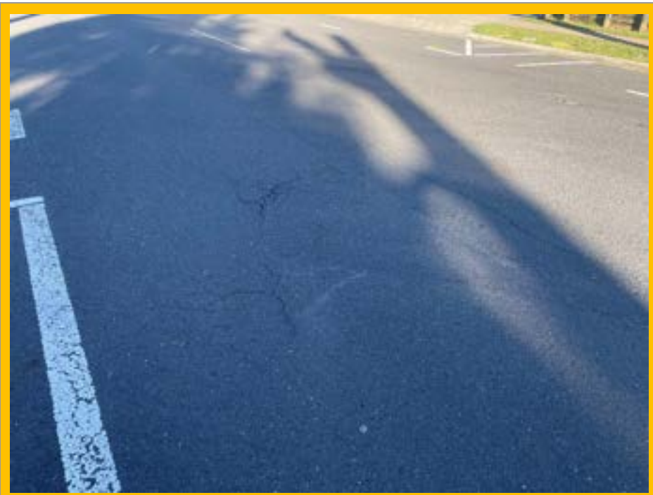
No. 036: cracking in surface at approx. 194, 195m
