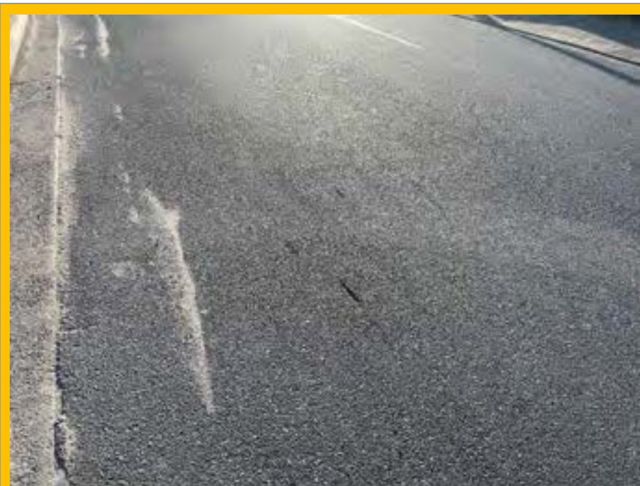
No. 006: general deterioration at 30m and beyond, and gouge marks at approx. 35m
