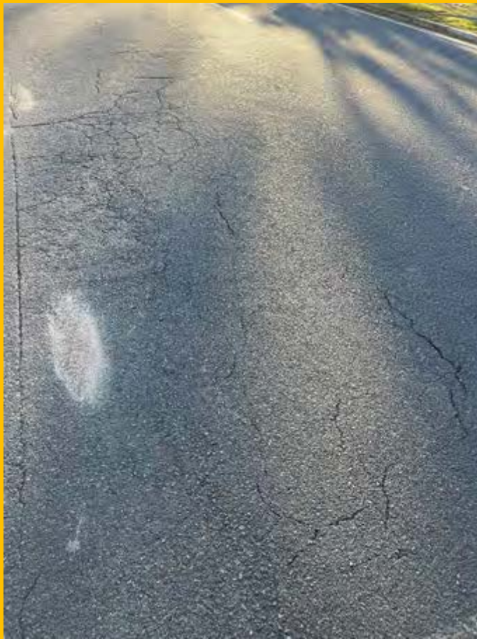
No. 041: deterioration and cracking to road surface from 190 to 193m at layback to 14 Harris St
