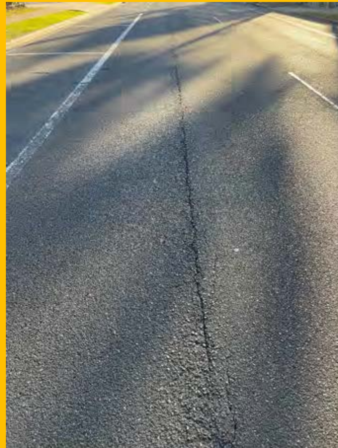
No. 084: continuation of crack in road joint materials
