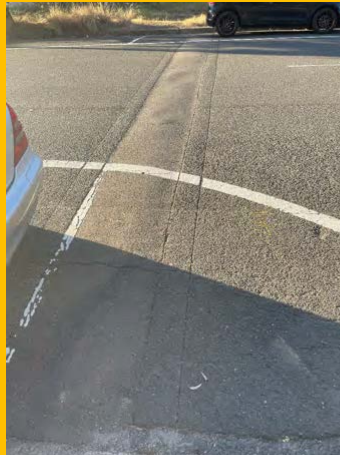
No. 120: cracking and repairs to road surface extending across full width of road at 491m
