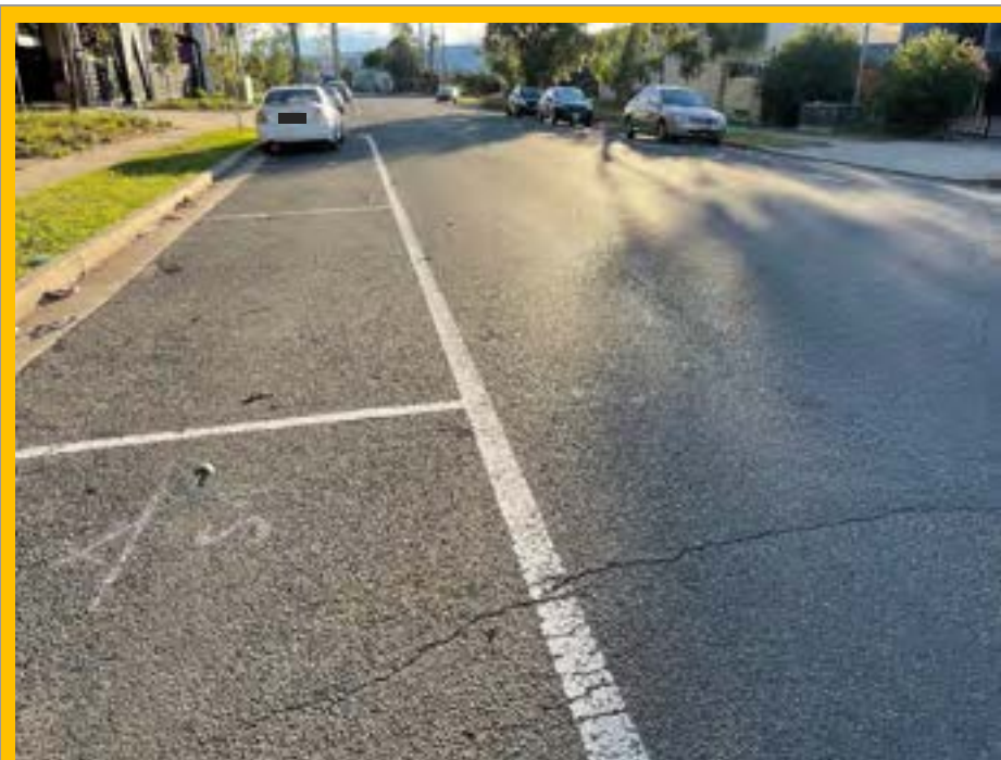
No. 110: 450m. lateral crack extends across full width of road
