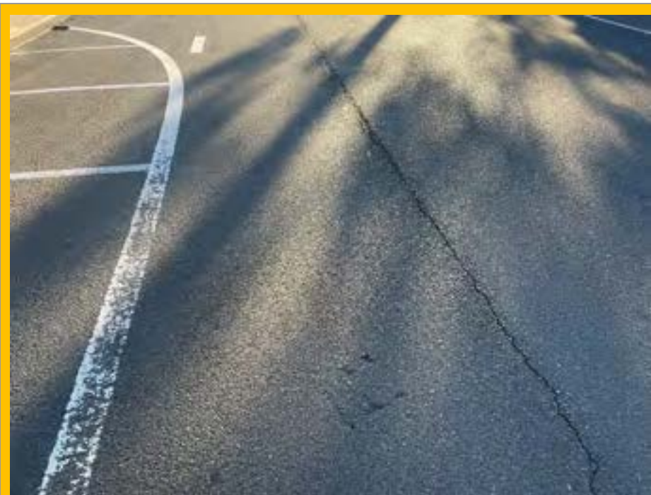
No. 059: continuation of crack and gouging in road surface at approx. 265m
