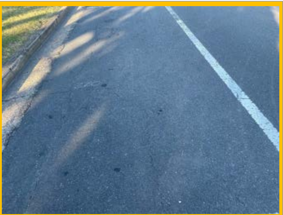
No. 050: cracking in surface from approx. 279m to 283m
