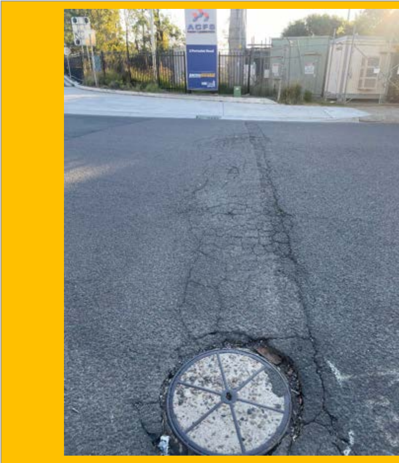
No. 001: Deterioration to road surface from intersection to Harris Street across full width of Forrester Road, viewed from Harris St.
