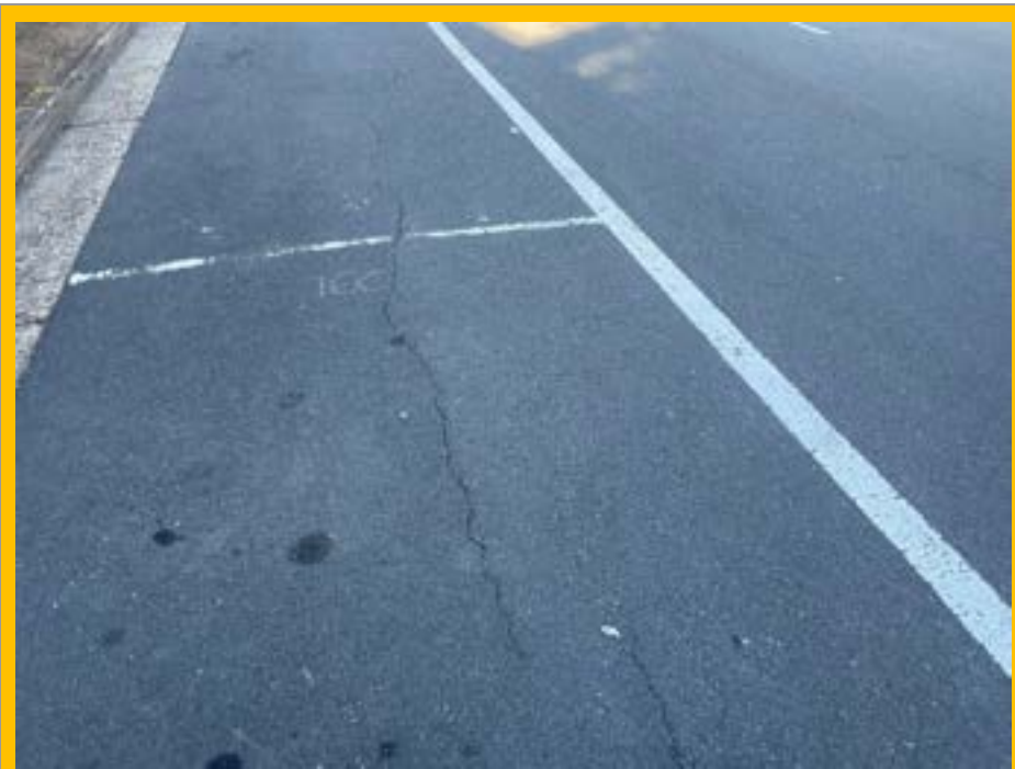
No. 028: Longitudinal cracking in road surface from approx. 158m to 163m
