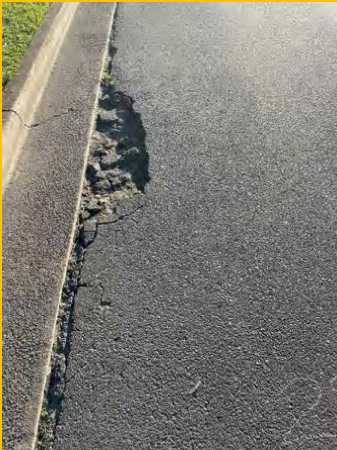
No. 067: Damage to road surface at kerb line
