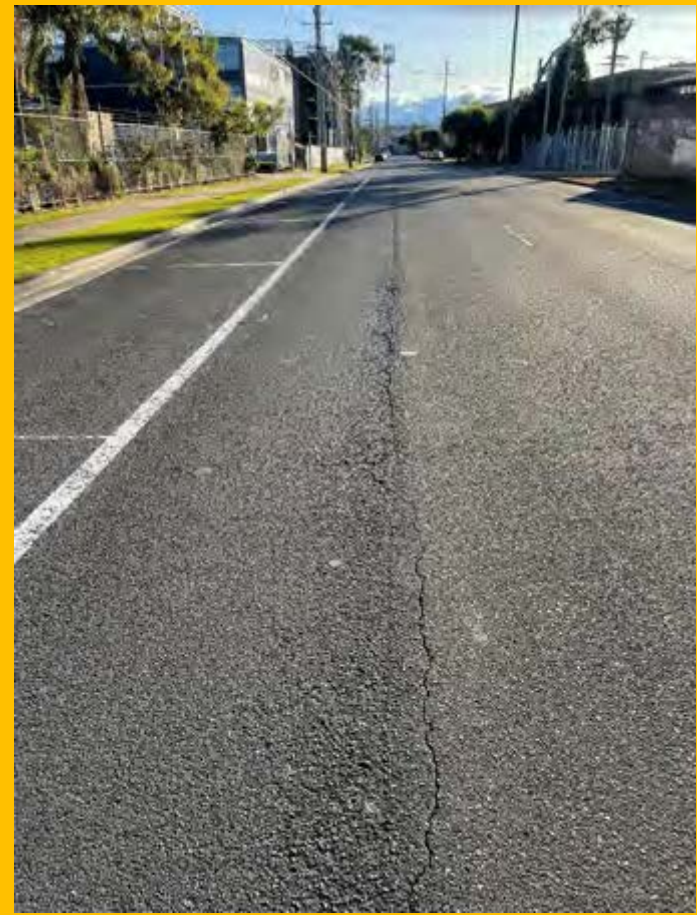
No. 074: cracking in road joint materials commences at approx. 297m
