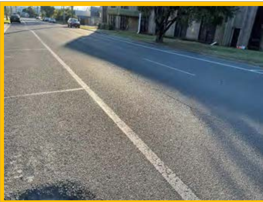
No. 101: crack in road joint materials
