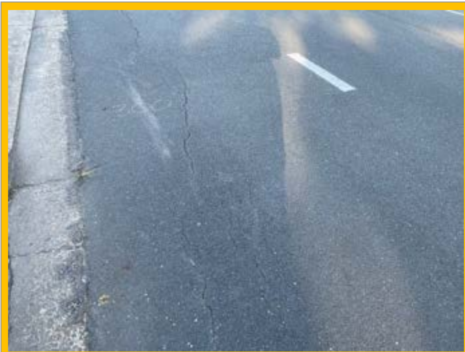
No. 055: longitudinal cracking from 298m to 310m
