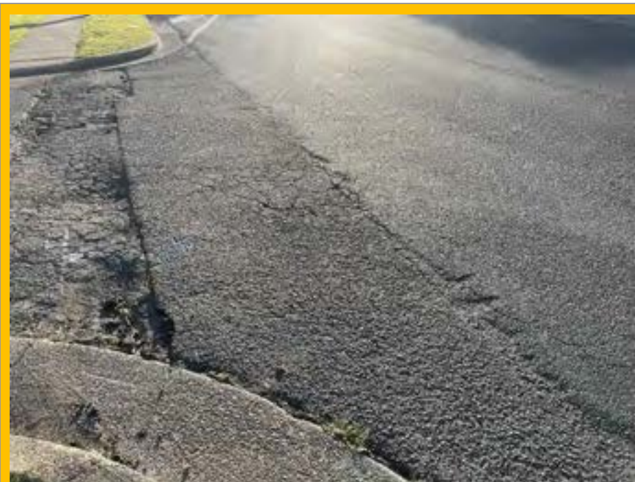
No. 095: deterioration of road surface repairs
