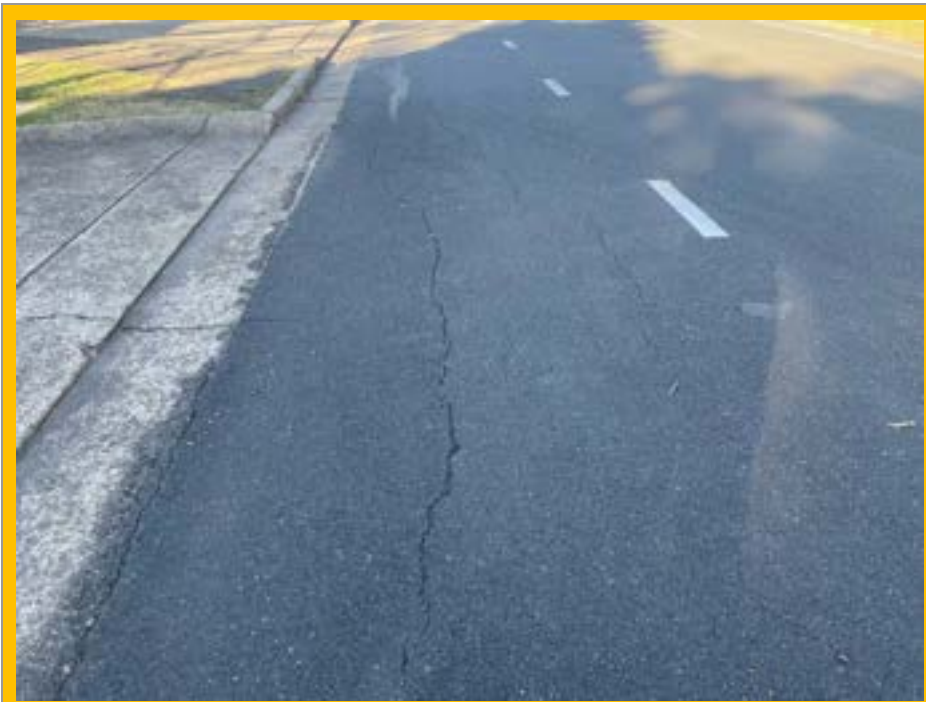
No. 057: longitudinal cracking and damage at entrance to 19 Harris Street (from 298m to 310m)
