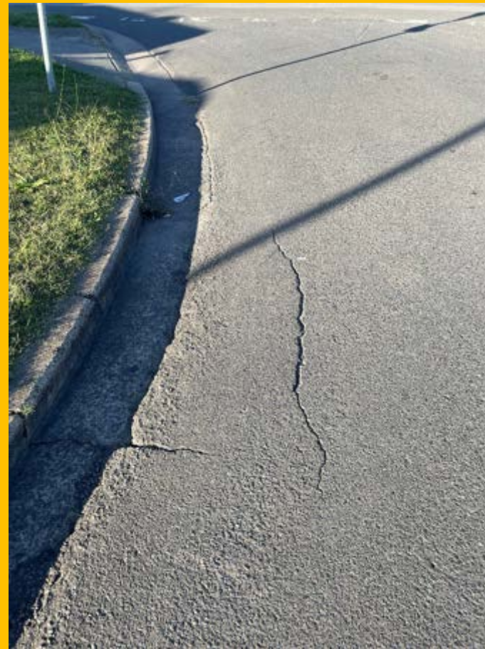
No. 090: Cracking and damage to kerb line at corner at approx. 545m
