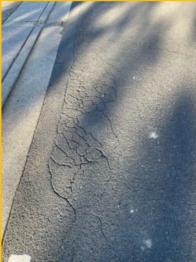
No. 067: damage to road surface at layback to 17 Harris St (356m to 364m)
