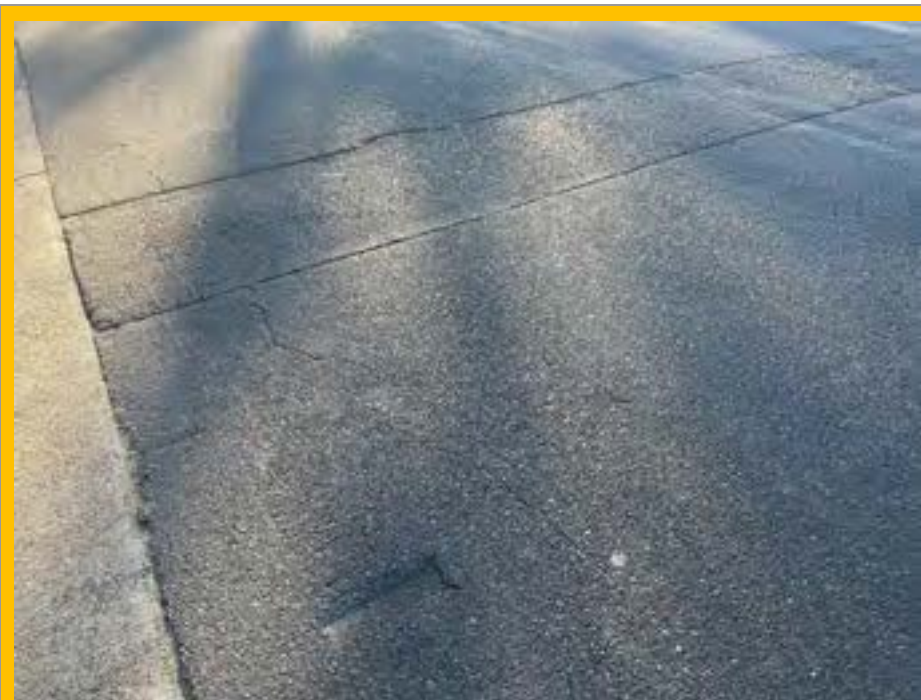
No. 014: repairs to road surface across width of street at approx. 78m
