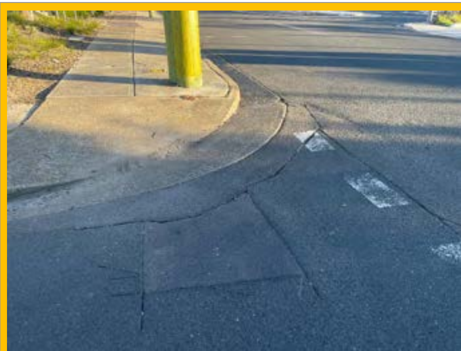
No. 129: depression and cracking to road surface at joins in road materials for previous repairs
