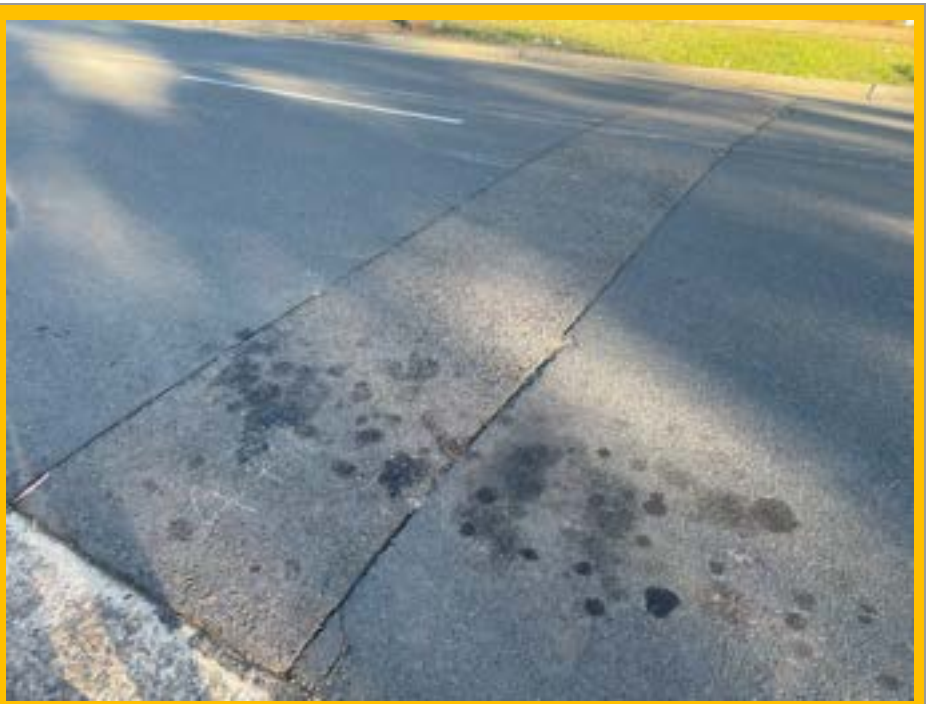
No. 082: Repairs to road surface across width of street at approx. 474m
