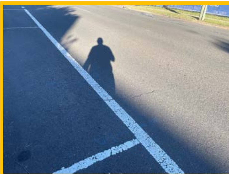
No. 031: Lateral cracking from the kerb toward the centre of the road at approx. 168m
