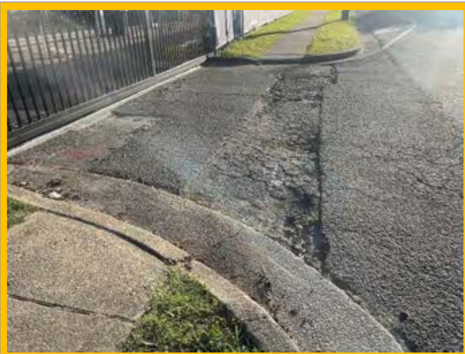
No. 094: significant damage to car park entrance
