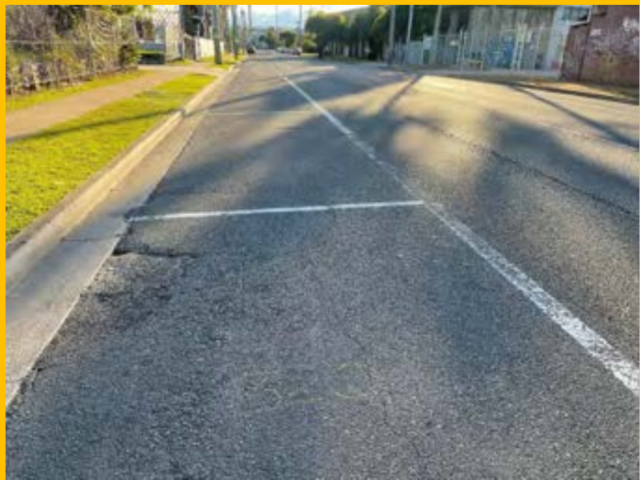
No. 082: 320m. continuation of parking bay surface cracks
