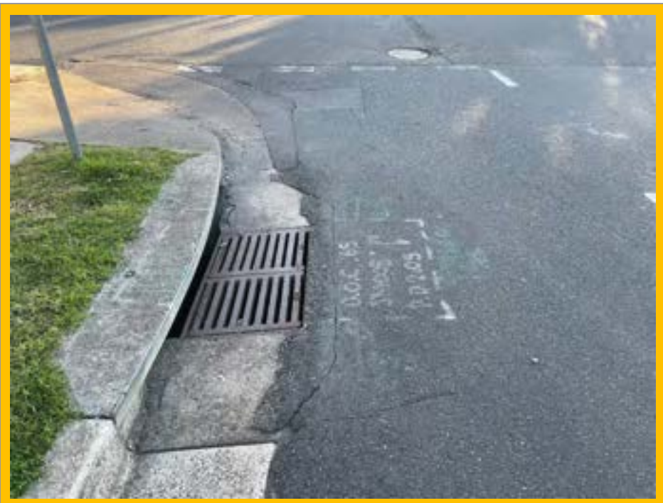
No. 128: cracking to road surface parallel to stormwater drain and at joints in road materials for previous repairs
