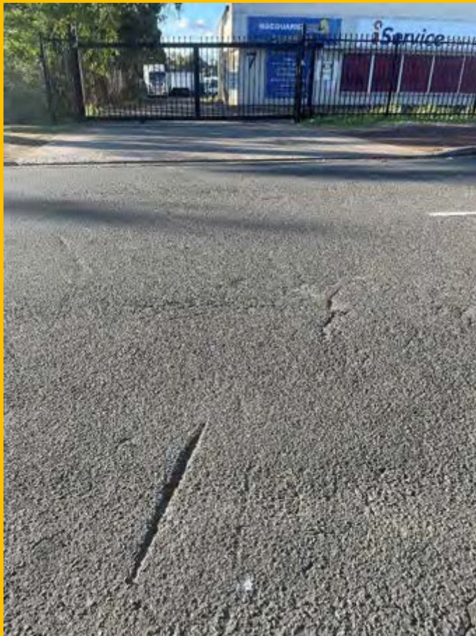
No. 023: multiple gouge marks and cracking at approx. 104m
