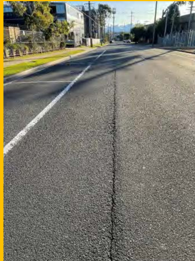
No. 080: continuation of crack in road joint materials
