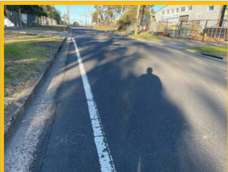
No. 063: 340m. lateral cracking at approx. 341m
