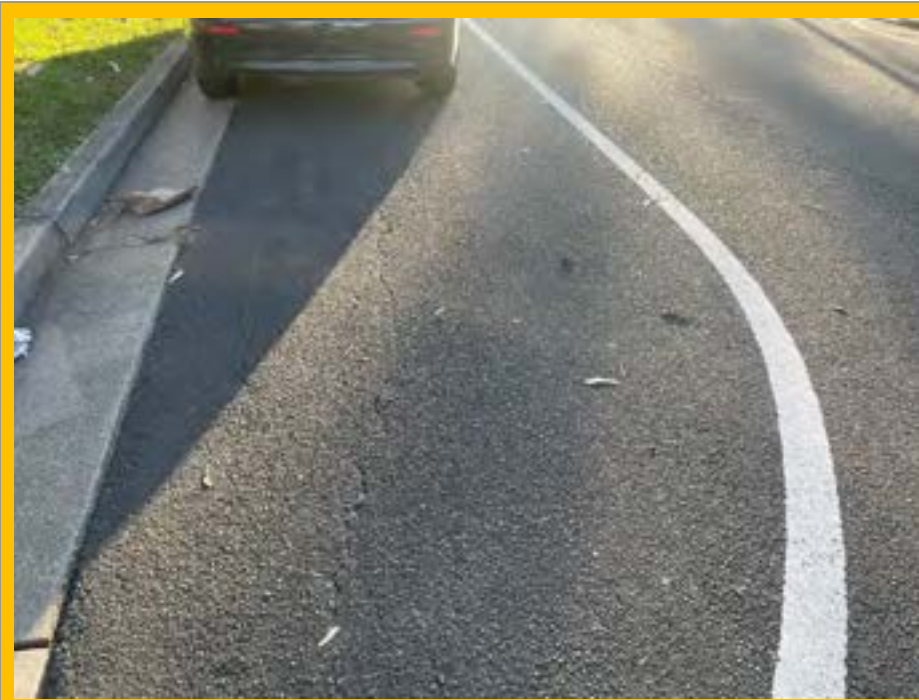
No. 107: deterioration of road surface in parking bays at 436m
