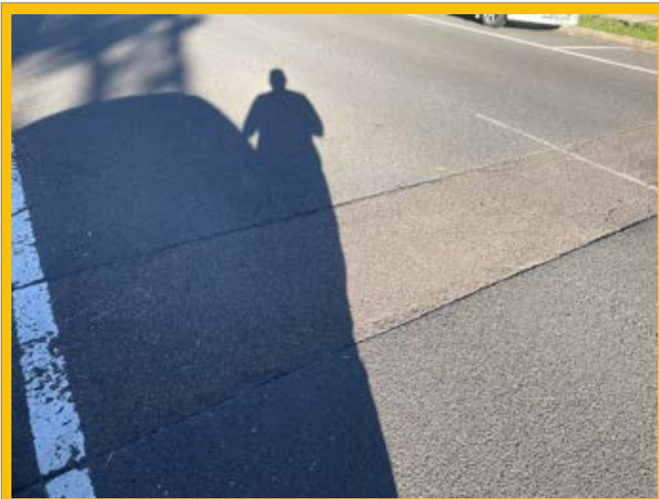
No. 017: Repairs to road surface across width of street at approx. 78m
