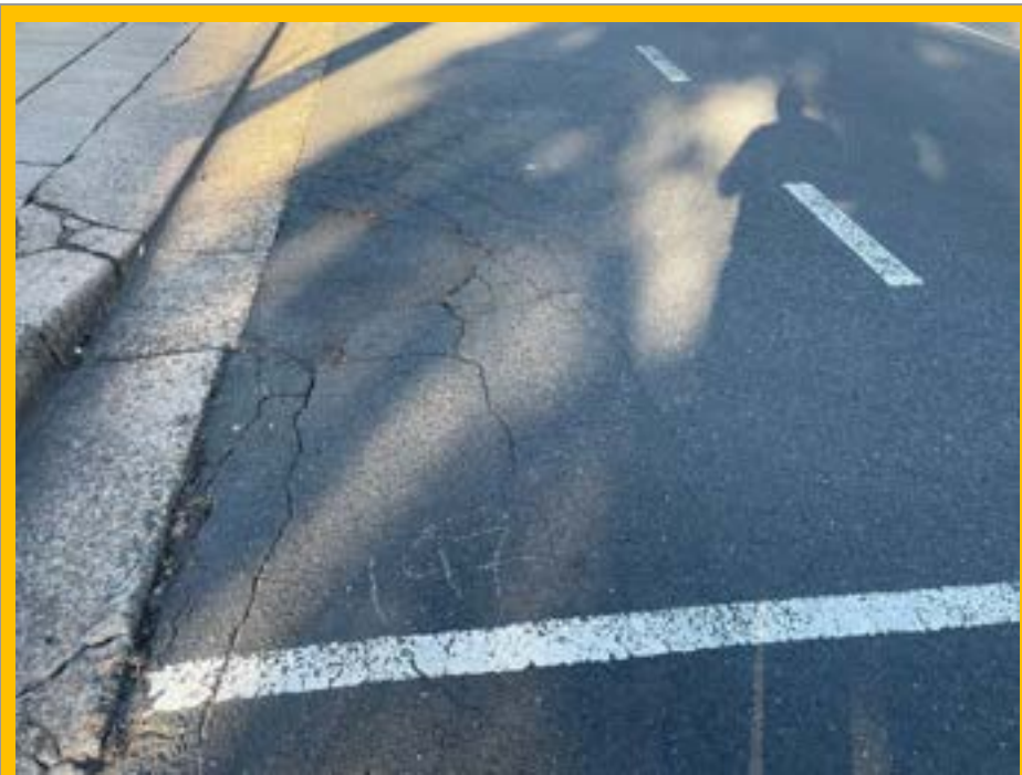
No. 037: damage radiating out from the layback at entrance to 21 Harris St (197m)
