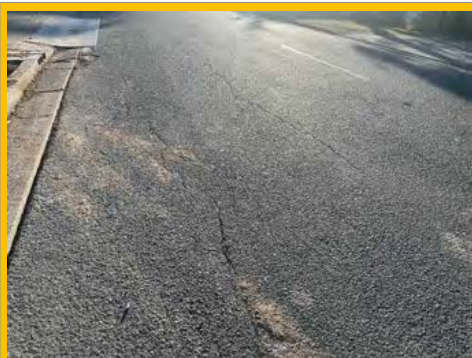
No. 019: multiple longitudinal cracks from approx. 92m and beyond
