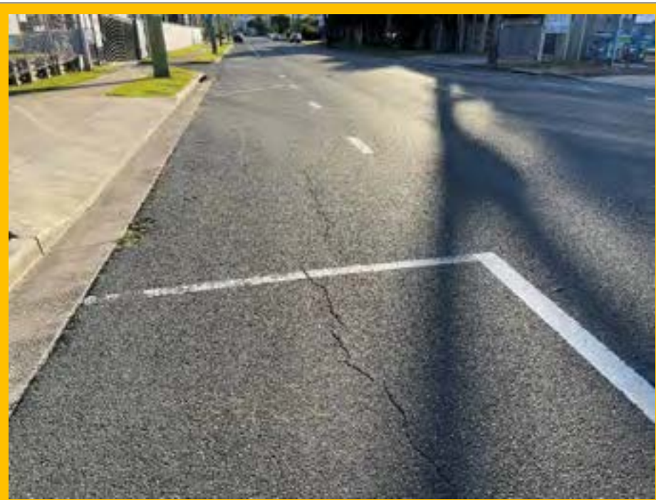
No. 088: 340m. continuation of parking bay surface cracks to 345m
