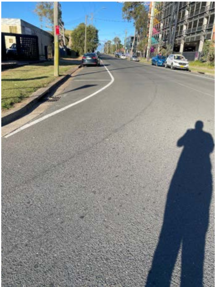
No. 001: Overview of Harris Street from the north-west corner at the intersection to Forrester Road. Survey began from this corner at 10m intervals, which are marked for distance reference.
