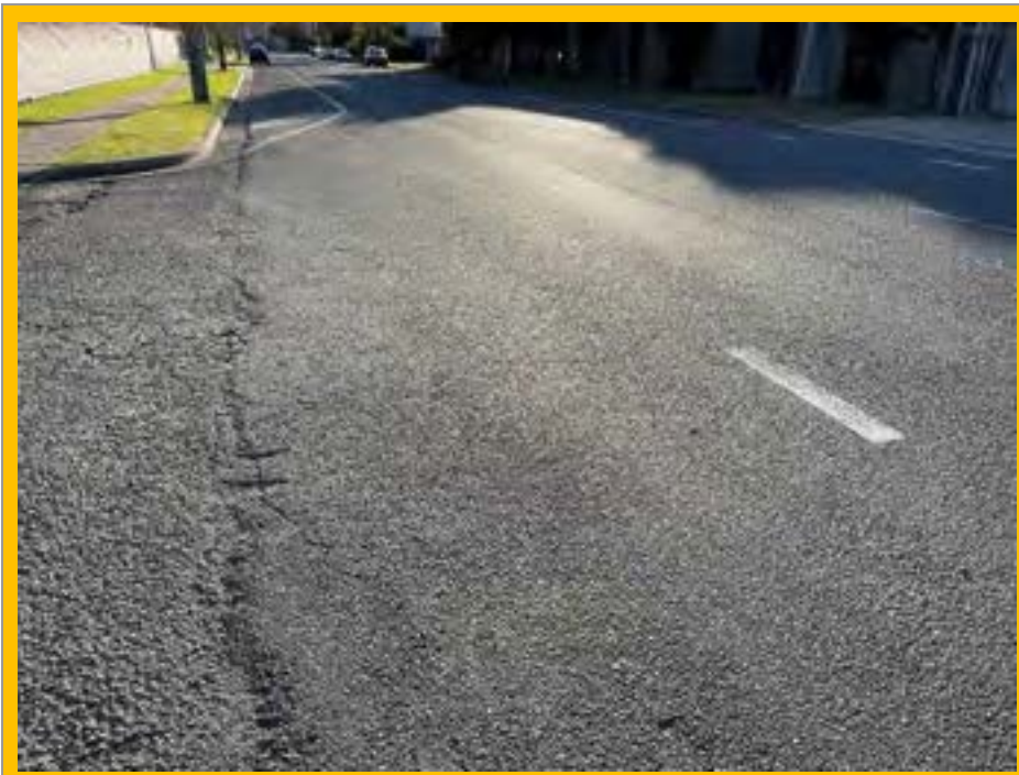
No. 093: 360m. Deterioration from the joint in materials leading to car park
