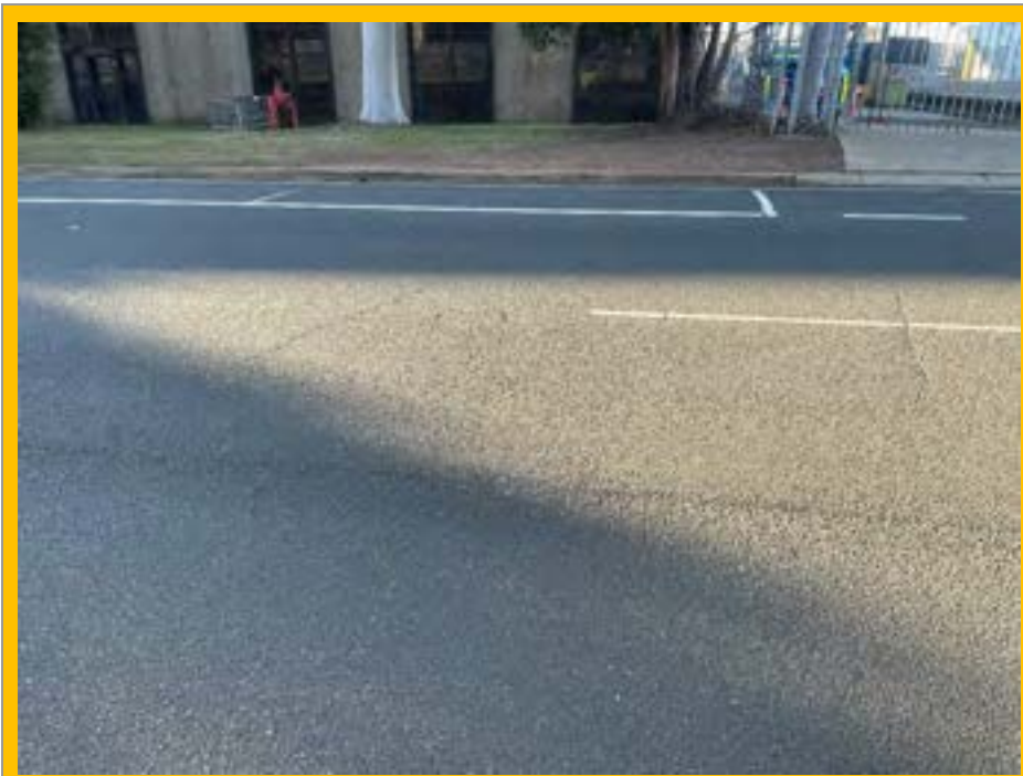
No. 097: lateral cracking to road centreline at 375m
