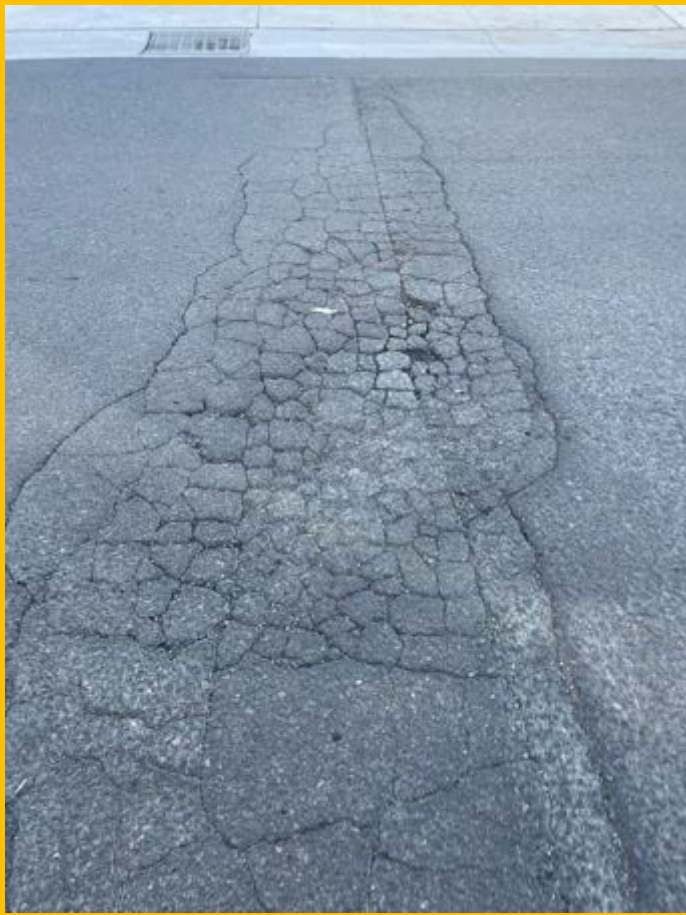
No. 005: deterioration and cracking of previous repairs to road surface
