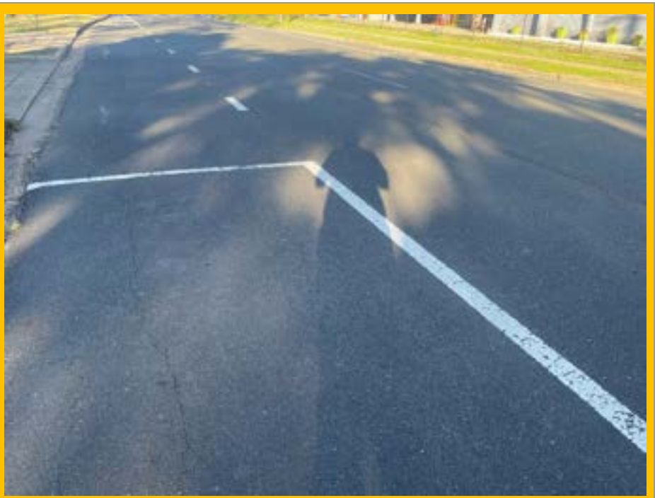
No. 054: longitudinal cracking from 293m to 300m
