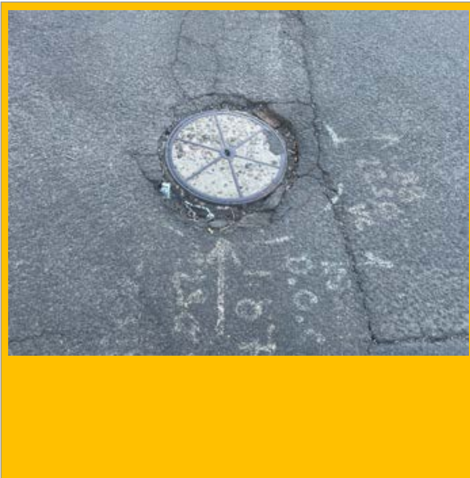
No. 003: damage to road surface at manhole cover
