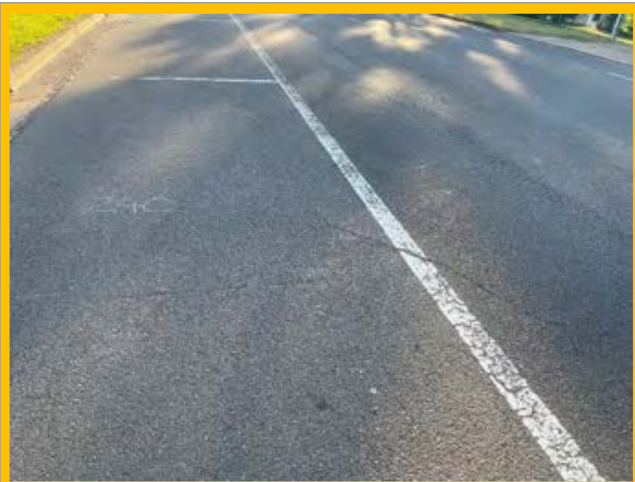
No. 050: cracking to road surface at 239m
