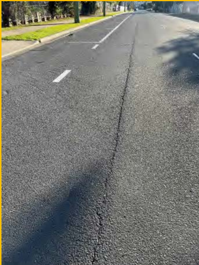
No. 063: continuation of crack in road centre
