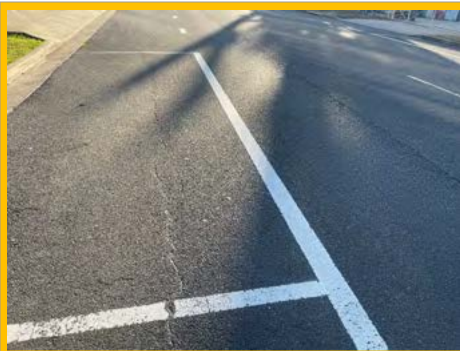
No. 087: continuation of parking bay surface cracks
