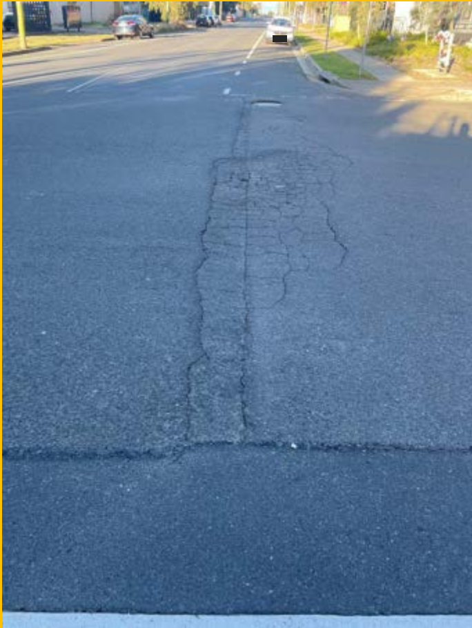
No. 002: Deterioration to road surface from intersection to Harris Street across full width of Forrester Road, viewed from ACFS/Pacific National facility entrance (2 Forrester Rd)
