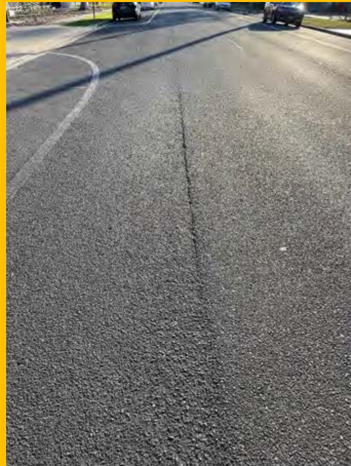
No. 104: crack commences at joint in road materials at 415m
