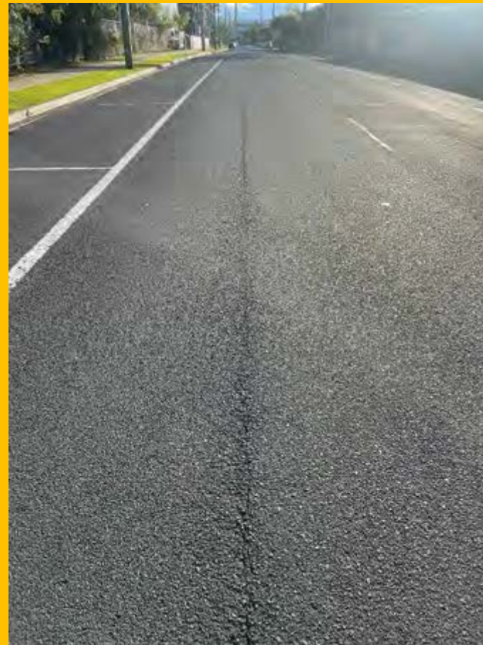
No. 068: continuation of crack in road centre
