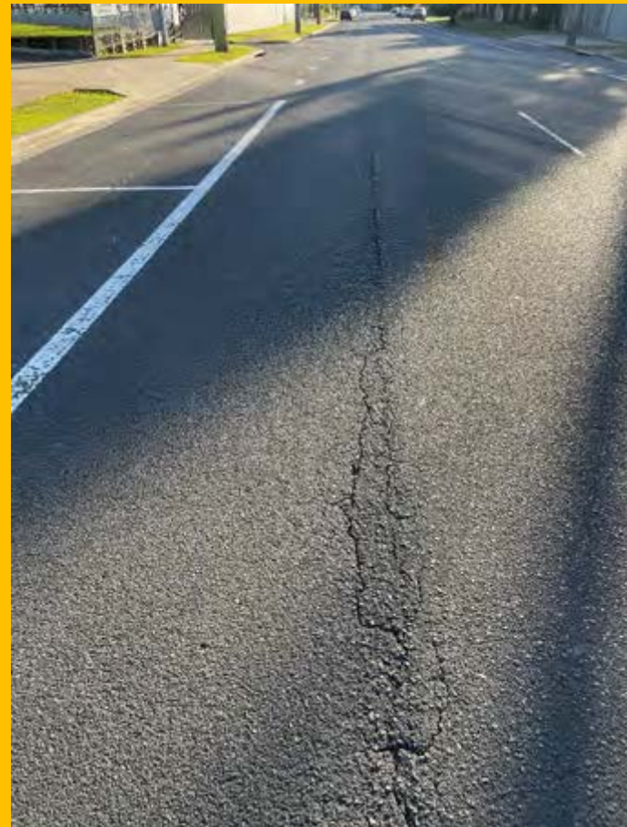
No. 086: continuation of crack in road joint materials
