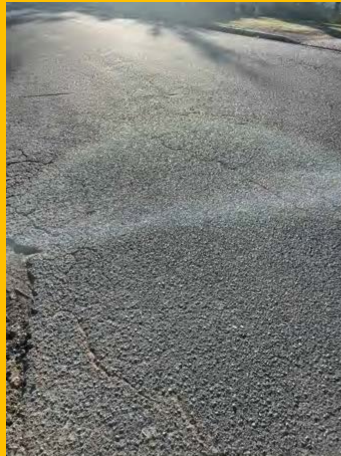
No. 022: continuation of cracking from 100m and beyond
