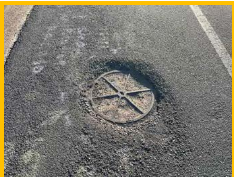
No. 100: depression at manhole cover at 395m
