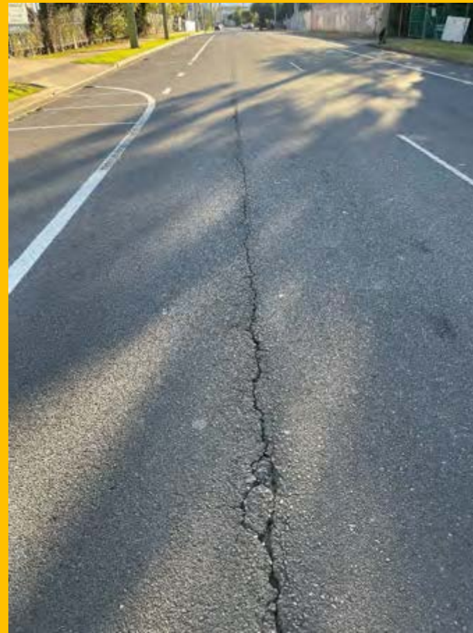
No. 058: continuation of crack in road centre
