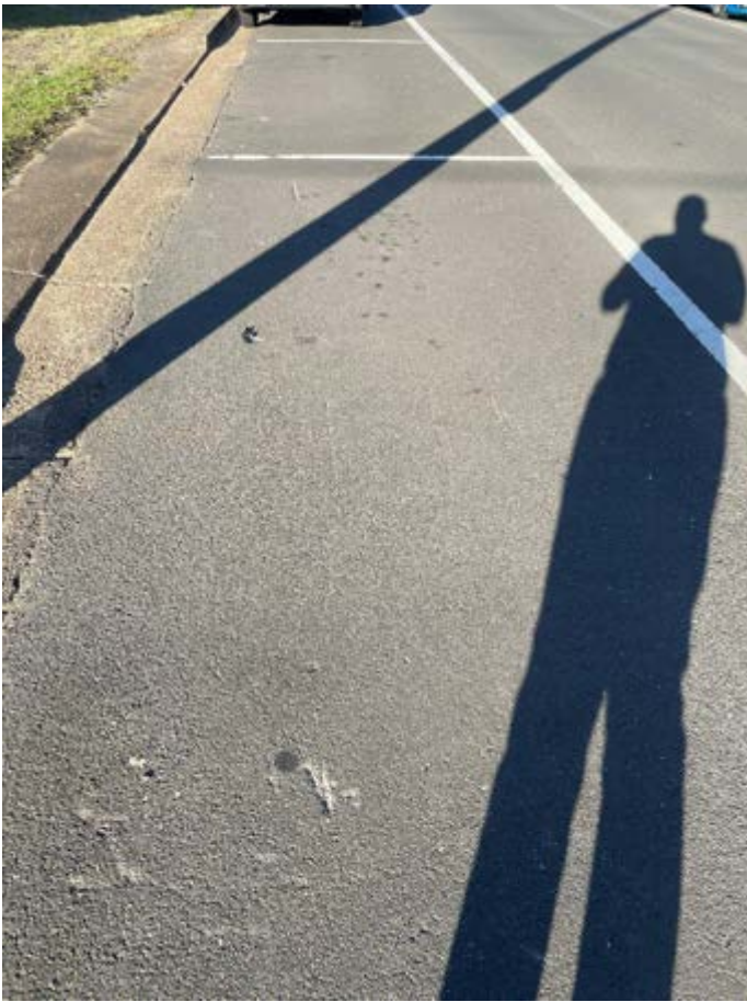
No. 005: Gouge marks on the road surface
