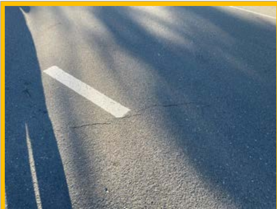
No. 059: lateral cracking at 315m
