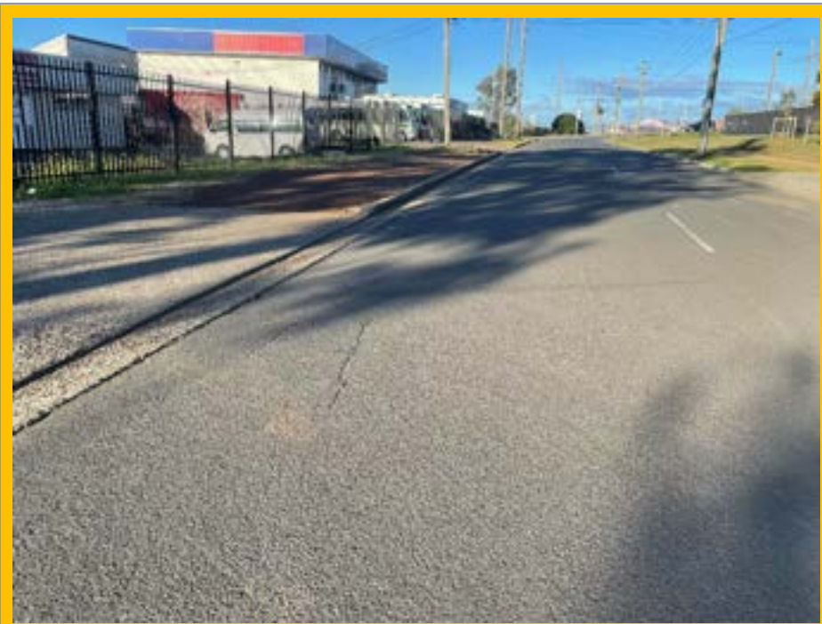
No. 077: cracking parallel to layback at 7 Harris St
