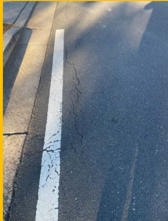
No. 066: continuation of cracking leading to driveway
