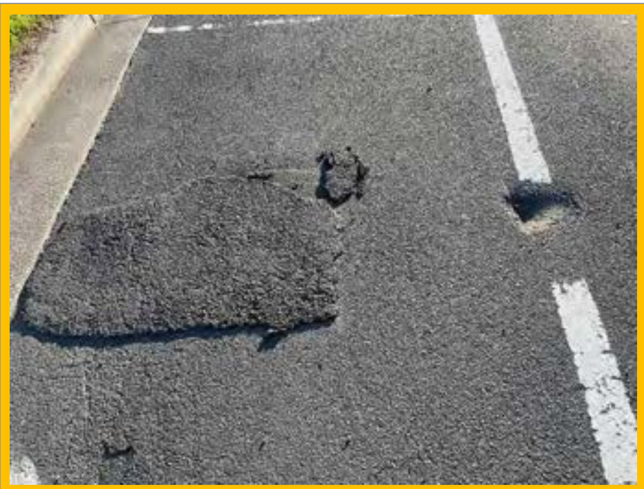
No. 048: road surface repairs and pothole at approx. 229m
