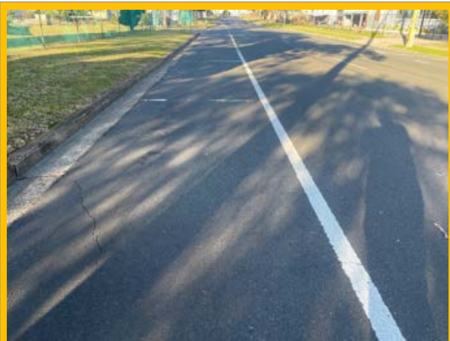
No. 048: cracking in surface at approx. 268m
