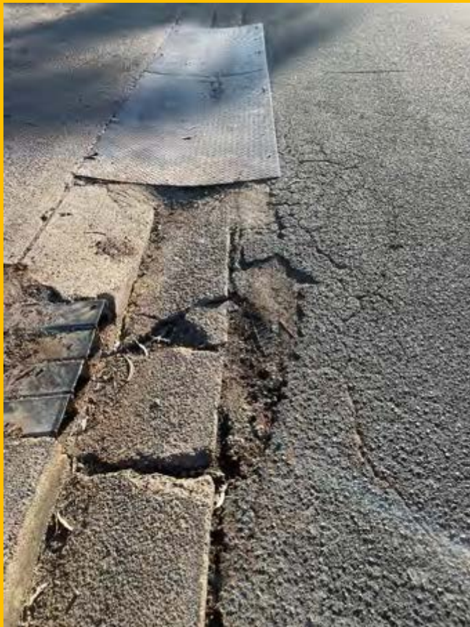
No. 021: damage at 6 Harris St
