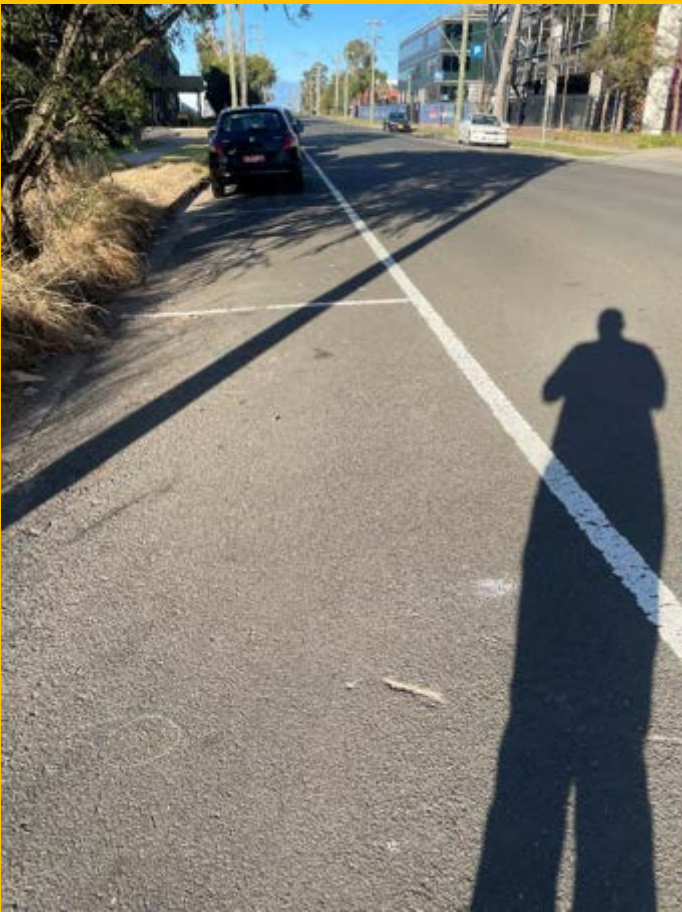
No. 012: 50m. Gouge marks to road surface
