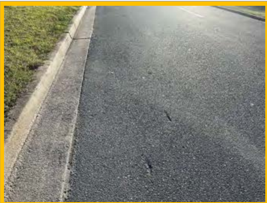
No. 008: gouge marks at 44m
