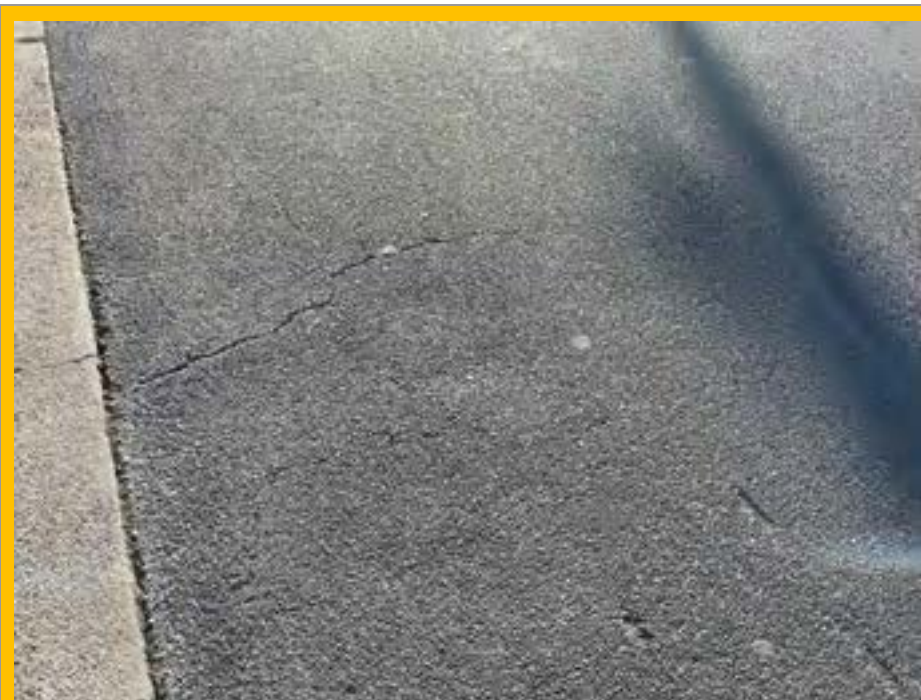
No. 011: lateral cracking extending from kerb line at 53m
