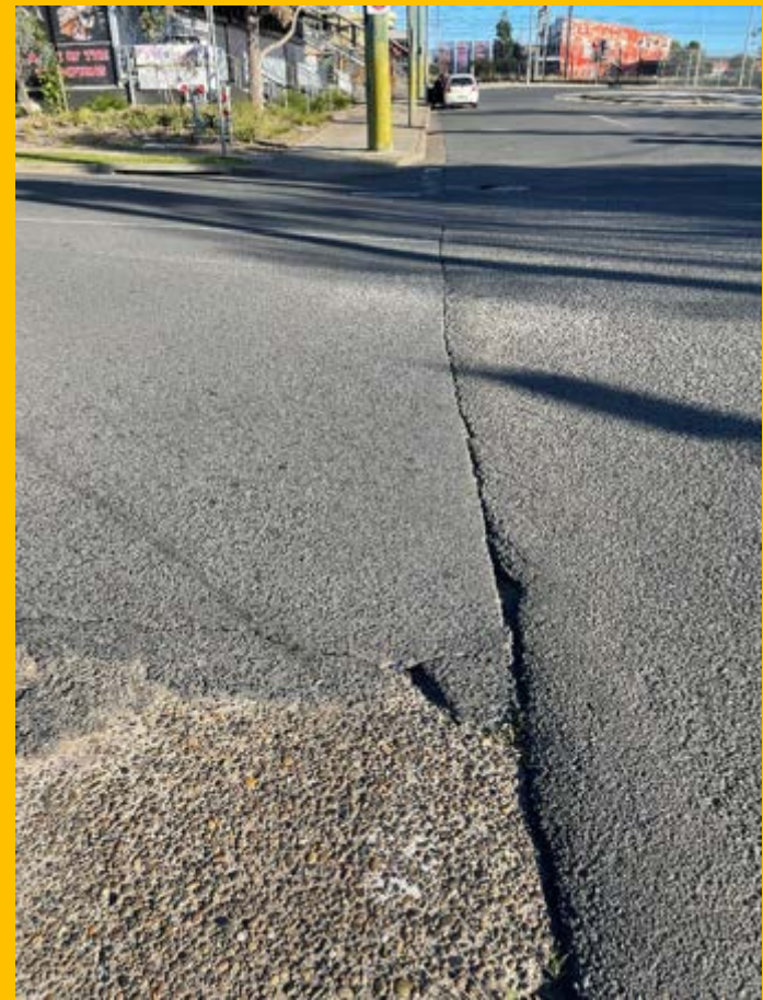
No. 002: Western end of Harris Street as it abuts Forrester Road. There is a crack at the join in road surfaces at this intersection and minor damage present.
