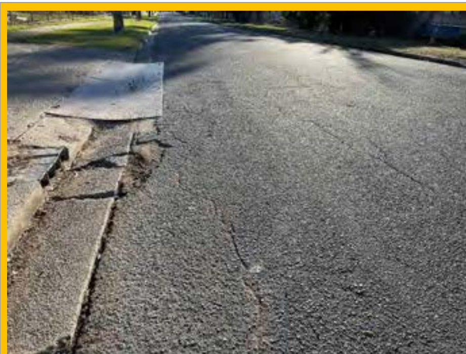
No. 020: 100m. continuation of cracking. Significant damage to road surface and layback at 6 Harris St
