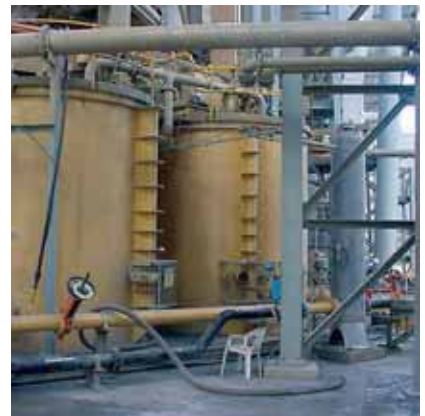
Callide Ash Handling Plant Modification
