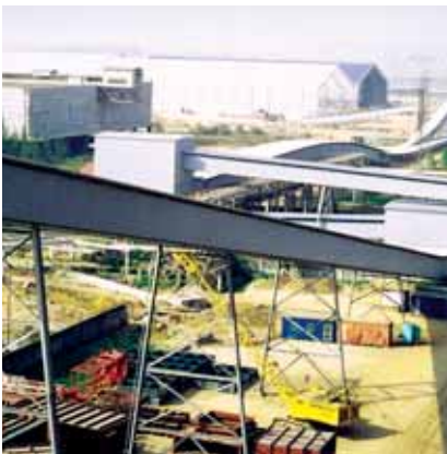
Pha Lai Coal Handling Plant
