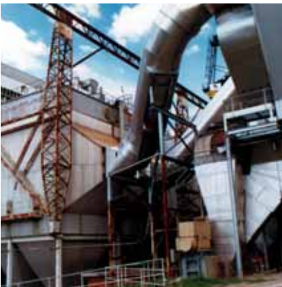
Swanbank Fabric Filter Plant
